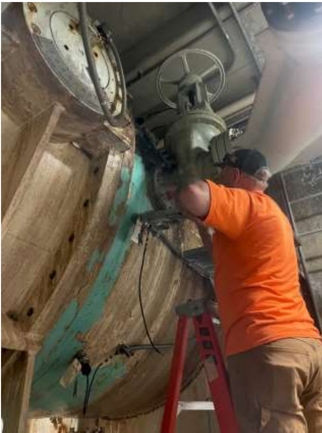
Accusonic Flow Meter Commissioning
