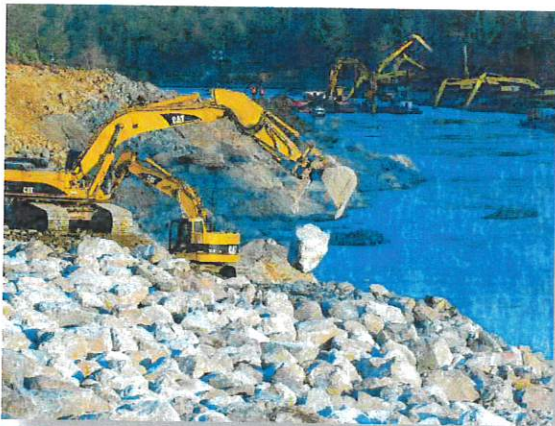
RSP - Oroville Dam Spillway Emergency Response
