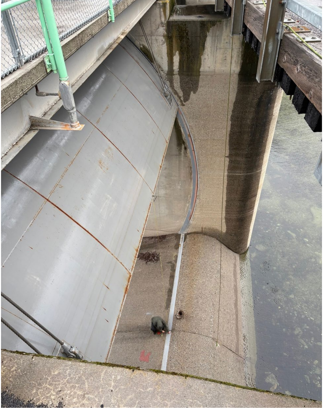
Beardsley Spill Gate at 25' Open
