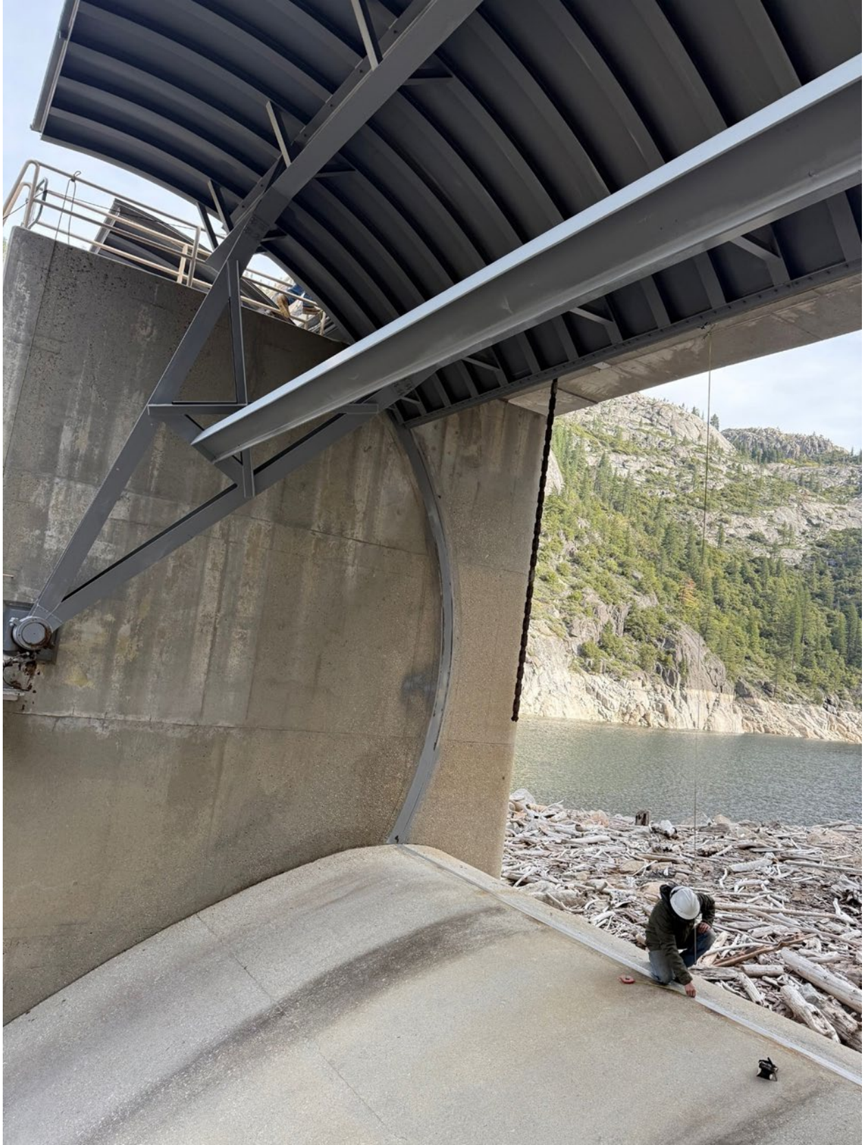
Donnells Spill Gate at 21' Open
