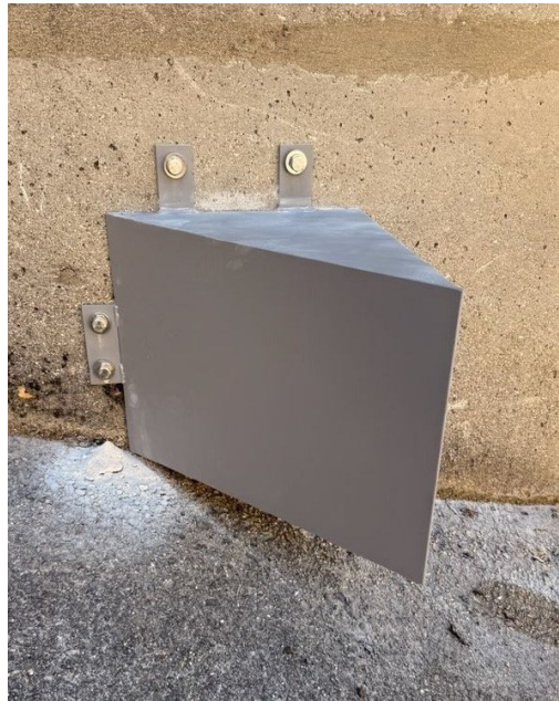
Drain Deflector DSOD Recommendation
